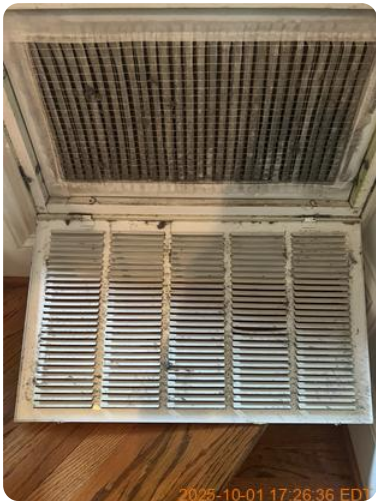
Air Conditioning/Filter 2025-10-01 17:26:36 35.20546150518853, -80.81630607476568 View Image
