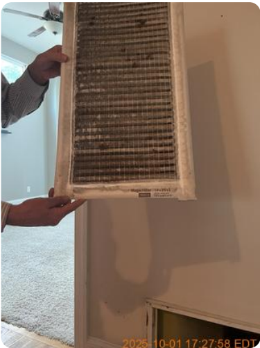
Air Conditioning/Filter 2025-10-01 17:27:58 35.20542119242018, -80.81625153670477 View Image
