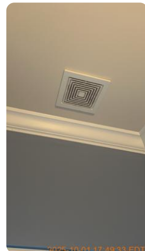
Exhaust Fan 2025-10-01 17:49:33 35.20547096542644, -80.81622092063365 View Image
